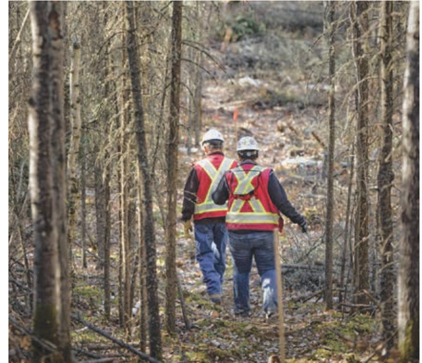
Surveying the right-of-way for the Northern Courier Pipeline, near Fort McMurray, Alberta. Our approach helps us to responsibly manage and minimize our environmental footprint in everything we do. That means we are always working to reduce our land disturbance, carbon intensity, energy consumption and water use throughout the life cycle of our assets.
